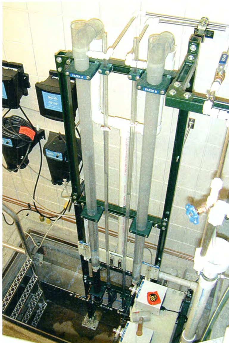
FIGURE A6. Sand filtration columns at DMWW pilot plant.
